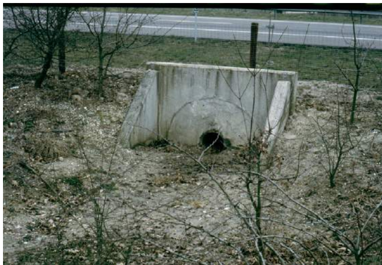
Fig. 7 Badger tunnel or underpass under Motorway A73, the Netherlands (photo Rob Jongman).
