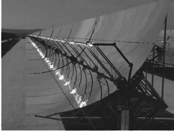
(a) Parabolic trough
