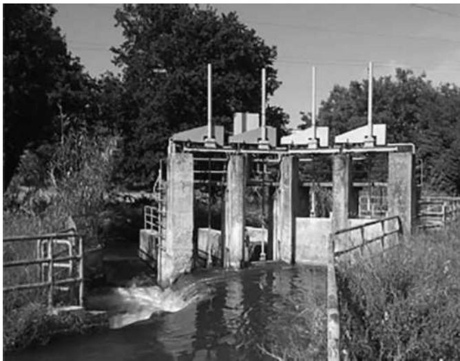
FIGURE 15 Example of fusegates: “Sant’Antonio I” IdroPower Station (Italy).
