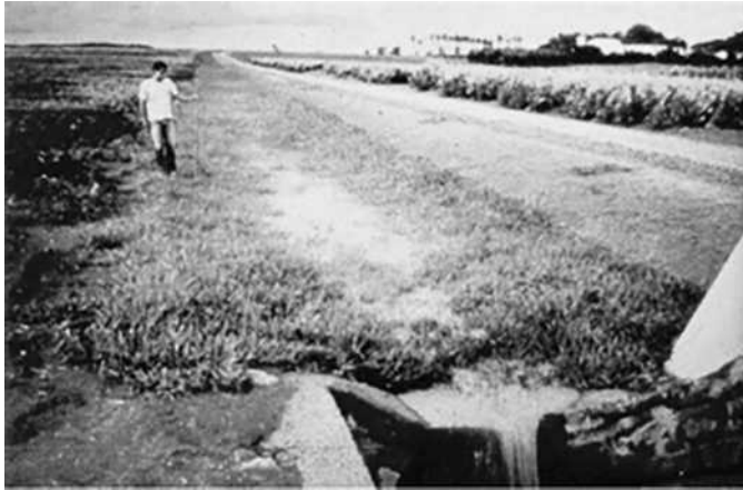
FIGURE 12 Grass waterway draining to a concrete drop inlet structure in southern Brazil. Source: Reichert and Cassol. [43]
