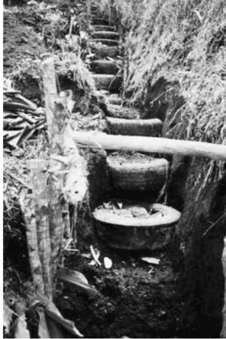
FIGURE 15 Gully stabilization with used tires, stones, and vegetation in Costa Rica. Source: Reichert and Cassol. [43]
