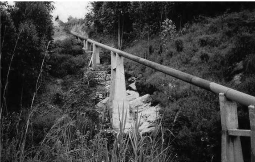
FIGURE 17 Example of a penstock.
