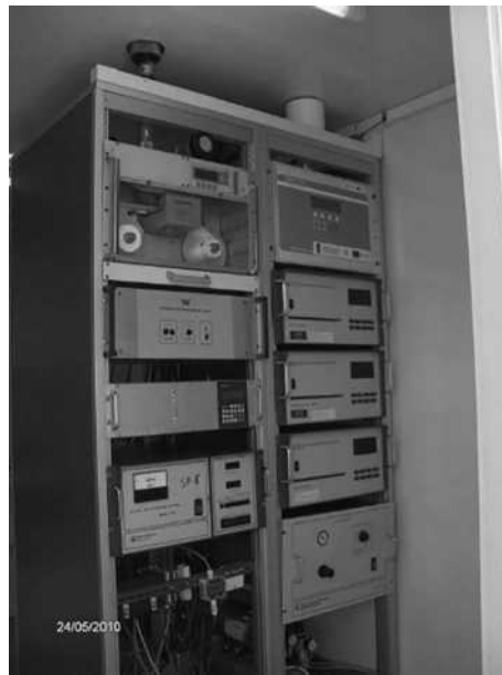
FIGURE 4 General view of an interior of a monitoring station.
