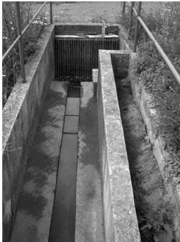
FIGURE 3 Mechanical pretreatment: screens and horizontal grit chamber. (Source: Photo courtesy of Jan Vymazal).
