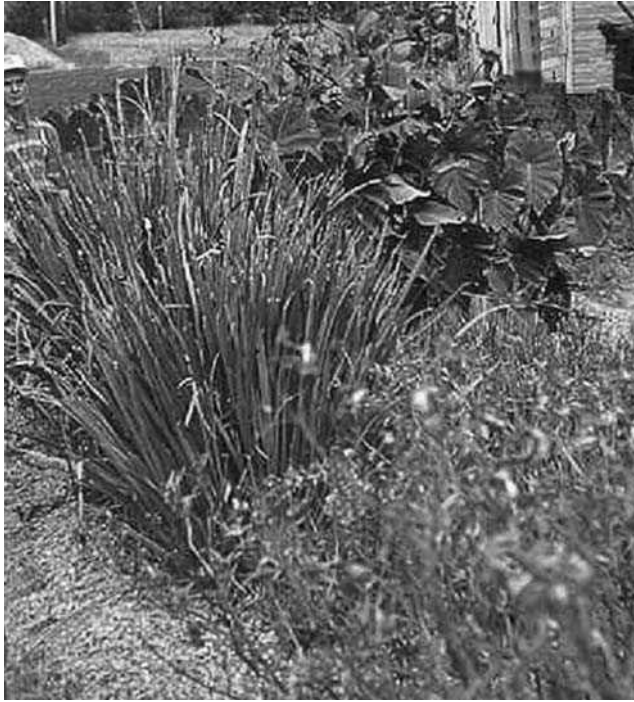
FIGURE 4 VSB wetland for treating onsite residential wastewater. This system uses gravel media and variety of wetland plants.
