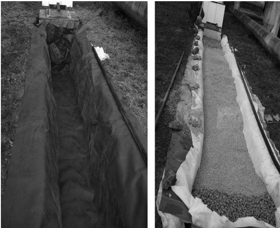
FIGURE 1 Constructed wetlands with horizontal subsurface flow. Left: filtration bed sealed with plastic liner, right: filtration bed filled with crushed rock with inflow and outflow zones filled with stones.
