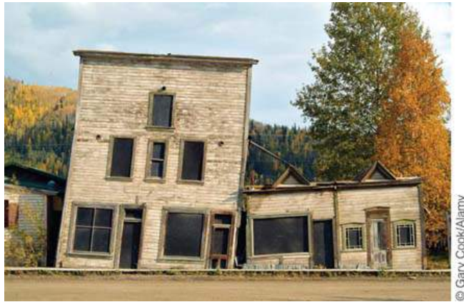
FIGURE 20.7 Thawing permafrost These buildings are sinking as the permafrost on which they were built thaws. Thawing permafrost causes ground subsidence, erosion, and landslides.
